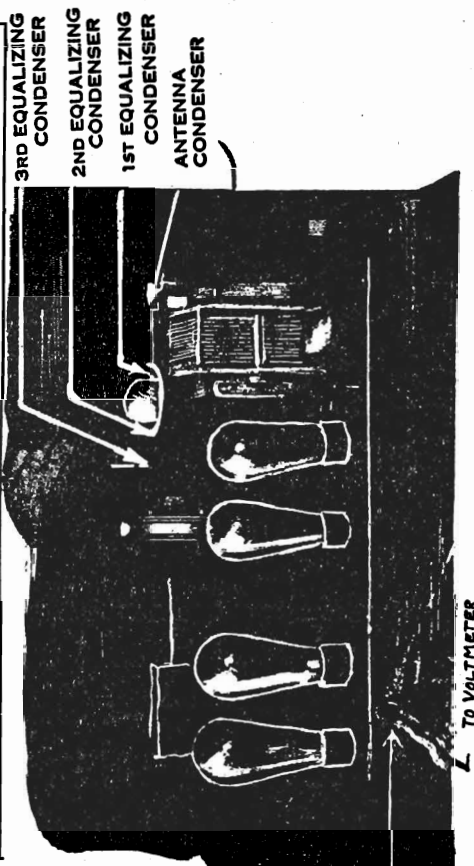
PHONE PLUG INSERTED APPROXIMATELY 3/4 OF THE WAY INTO THE JACK OR JUST FAR ENOUGH TO OBTAIN A READING OF APPROXIMATELY 15 VOLTS WITH NO SIGNAL TUNED IN
